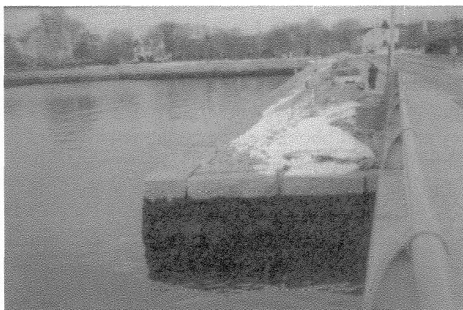
Recent repair work on this corner of the seawall on the Goat Island connector is a huge improvement over the corner's previous condition.
